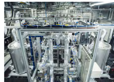
Equipment within the CO 2 Circulation Plant
