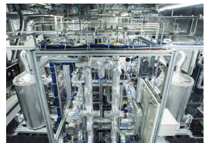
Equipment within the CO 2 Circulation Plant
