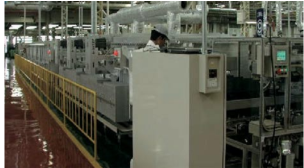
Fig. 13 Photo of the new energy-conservation-style brazing furnace
