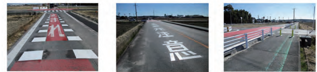
① Highlighted the "Stop" sign to remind pause ② To encourage slowdown, "Accident Warning" is displayed on the priority road ③ Newly installed "guard pipe bollards" to protect pedestrians
