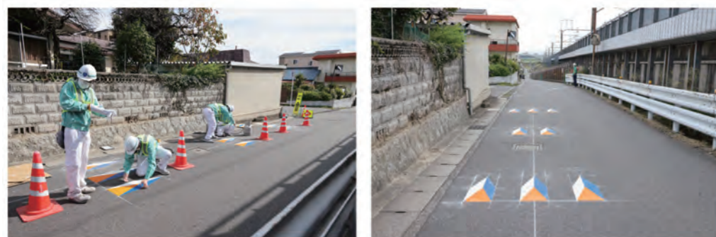
Fig. 9 Construction work to install road markings to encourage slowing down on the road along Shinkansen in Kandacho 3-chome
